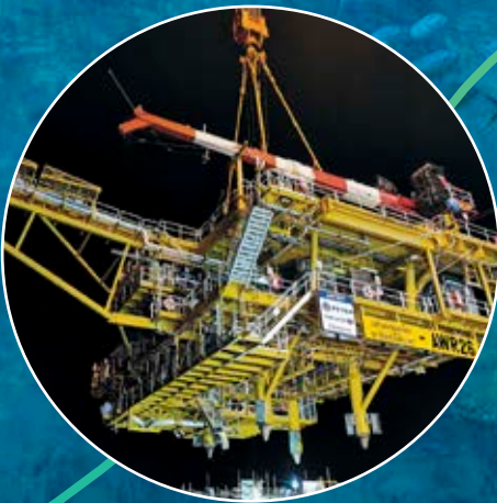
Relocation of Arthit Asset's wellhead platform topside for reuse to maximize resource efficiency
