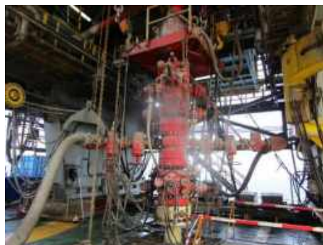
Fig. 11. Blowout preventer (BOP) stack linked to the rig
